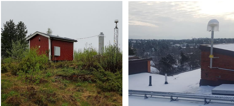
Figure 1: Left: Sveg is one of the Swepos class A stations. It has an old monument (established in 1993) as well as an additional monument (2011). Right: Gustavsberg is a Swepos class B station with a roof mounted GNSS antenna established mainly for network RTK purposes.
